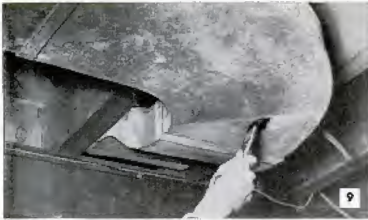
In time, rust will work through the protective galvanizing on ducts of the heating system. Aluminum paint is added protection
